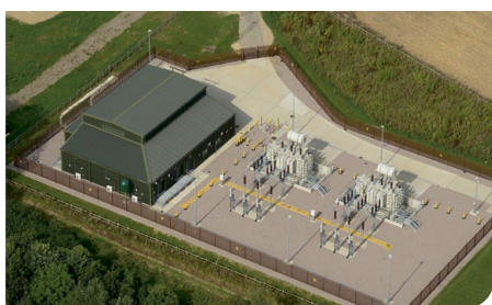
Onshore converter station at Salle, Norfolk
